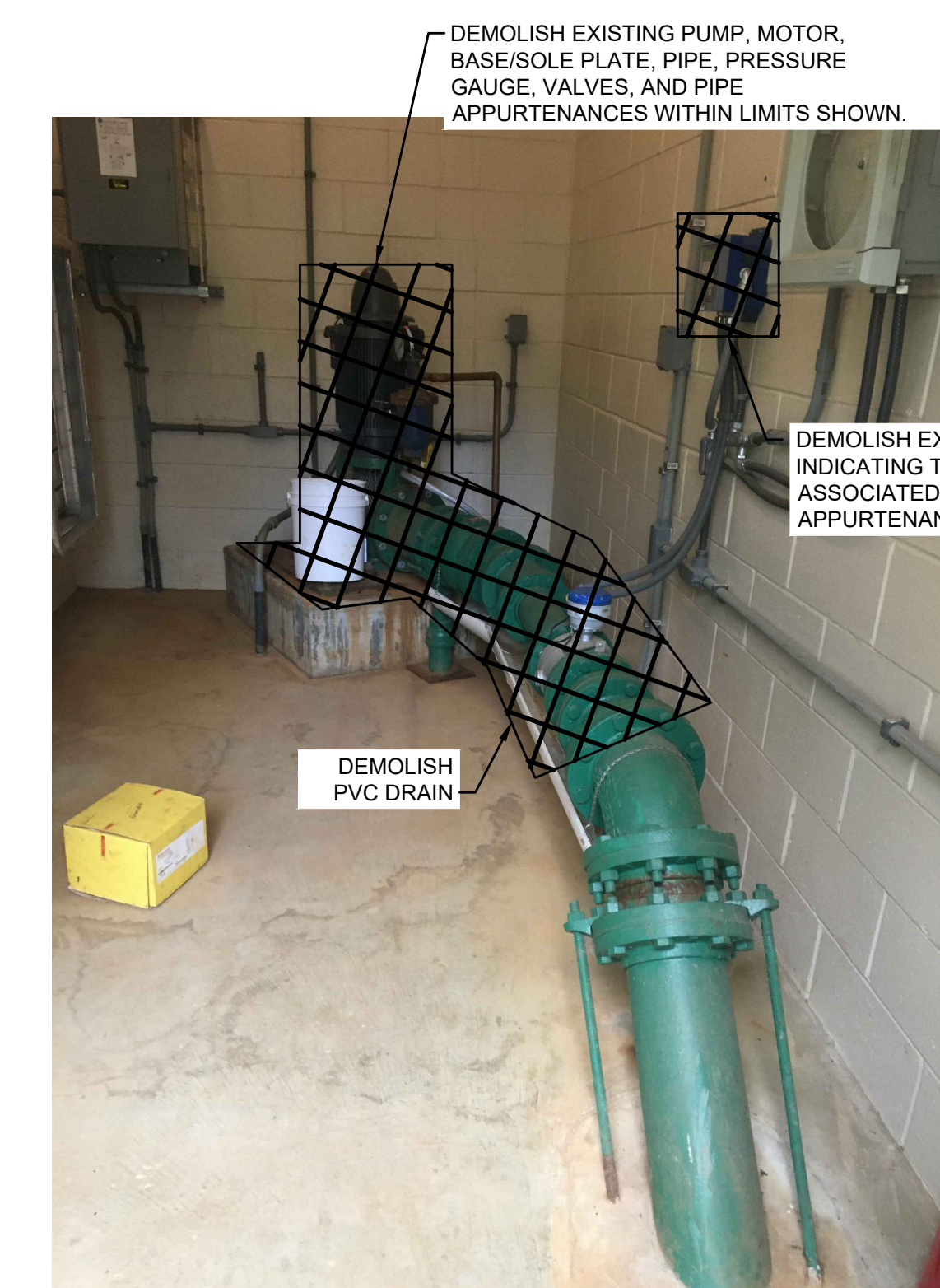
PHOTO 3 SCALE: N.T.S. WELL NO. 14 PUMP, MOTOR, AND PROCESS PIPING
