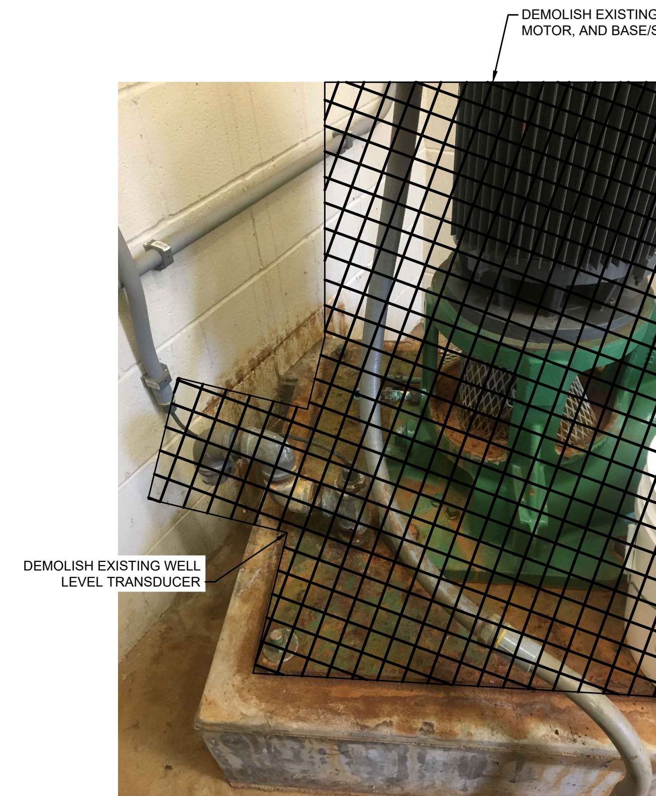
PHOTO 2 SCALE: N.T.S. WELL NO. 14 PUMP, MOTOR, AND LEVEL TRANSDUCER
