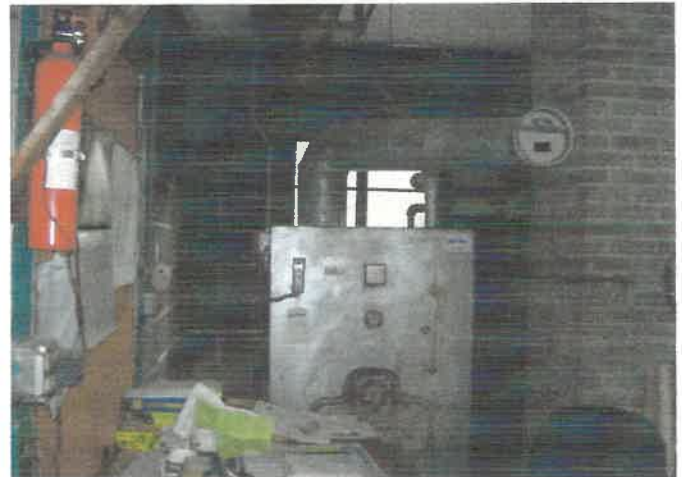
oil-fired steam boiler
