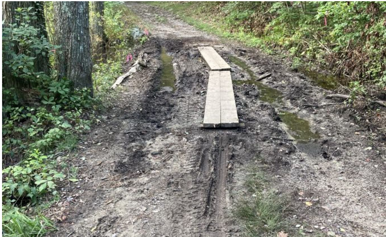
Photo #2: Closer view of the Project Area (inner 10-feet of the existing 14-foot wide fire road).
