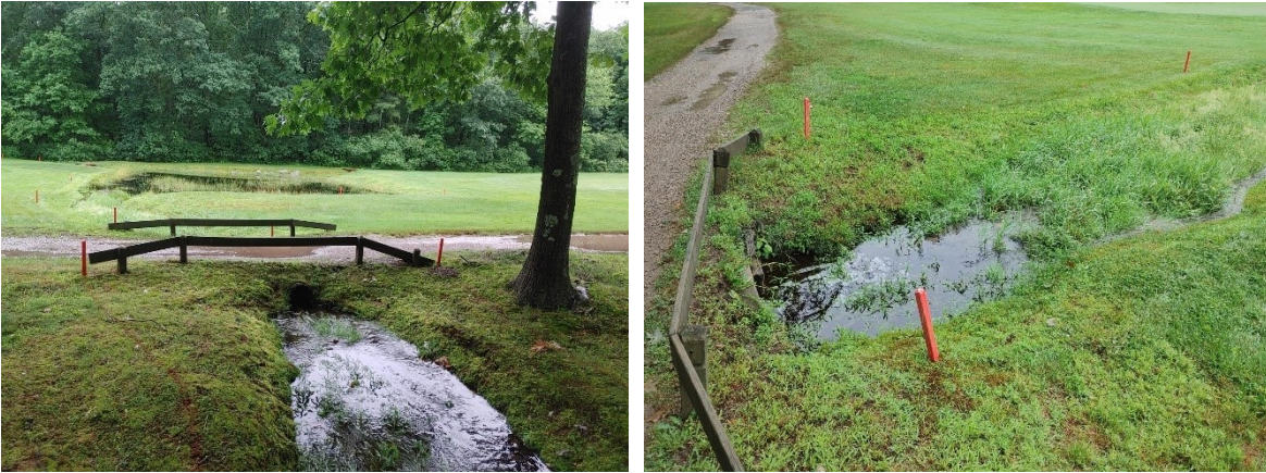
Left Photograph: View facing south of existing undersized culvert and subject pond.
