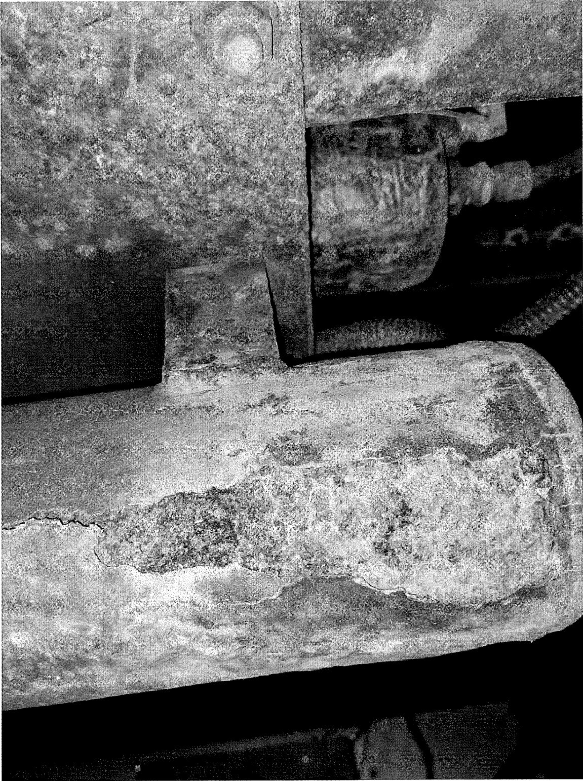
Figure 7- rotting quick recovery tanks
