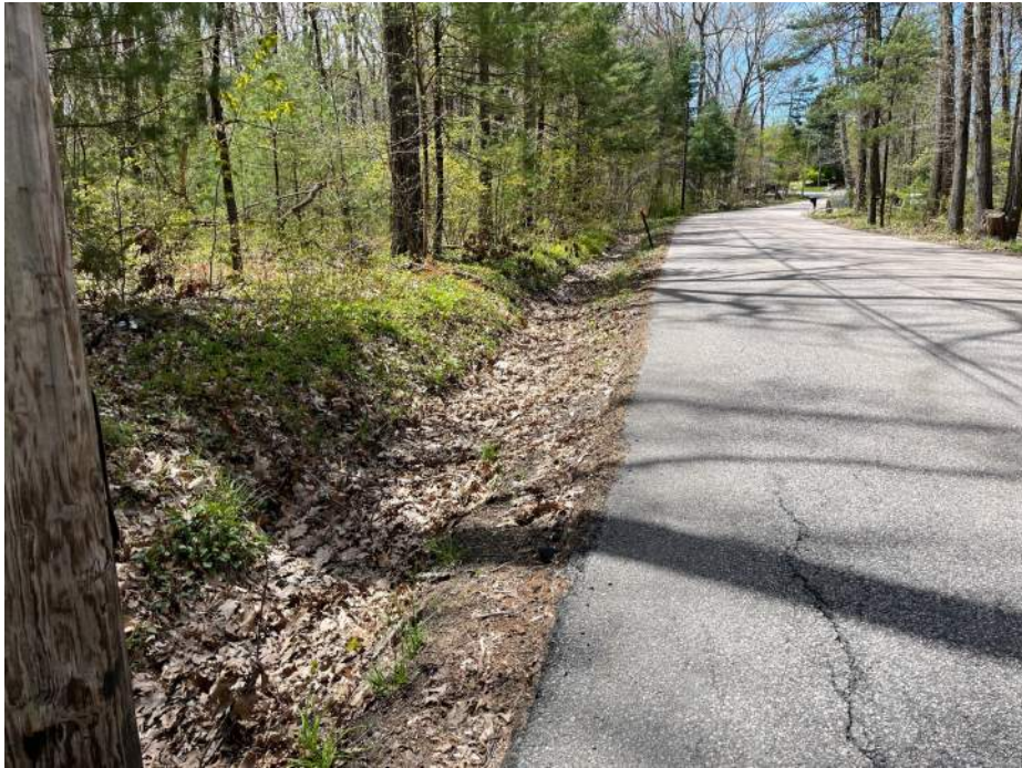
Photo 3: Non jurisdictional drainage swale (CH series) along south shoulder of Walnut Street.
