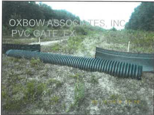
PVC Culvert "Gate"
