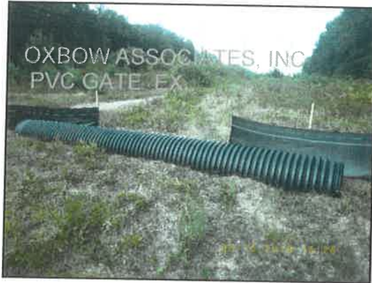
PVC Culvert "Gate"
