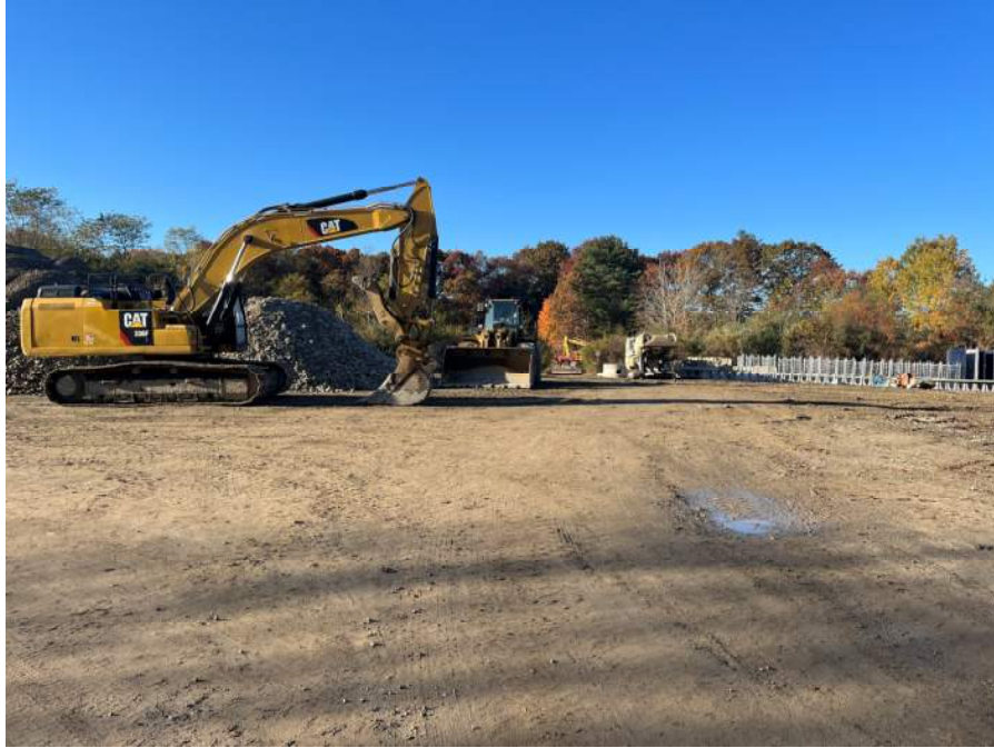
Photo 13: Central portion of development site, which has been cleared and graded under the former OOC.
