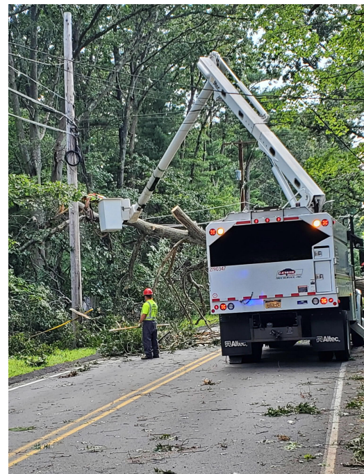
Downed power line from an intense storm on August 4, 2020
